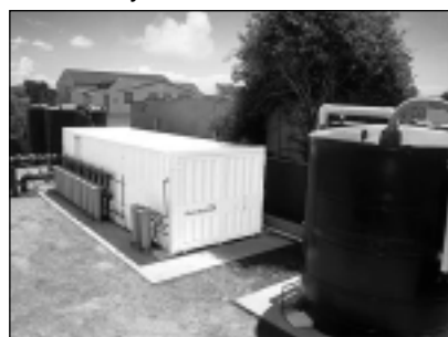
Basin Water perchlorate and nitrate removal systems
