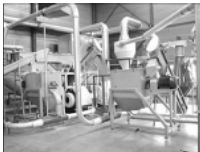
PHB installation for PS-ABS separation
