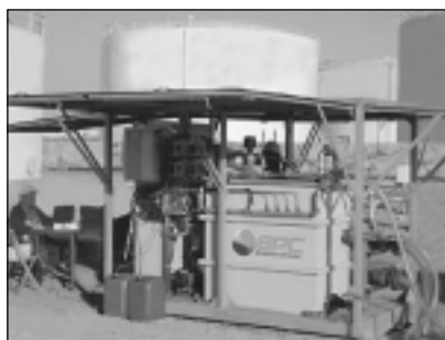
BPC's bioremediation unit
