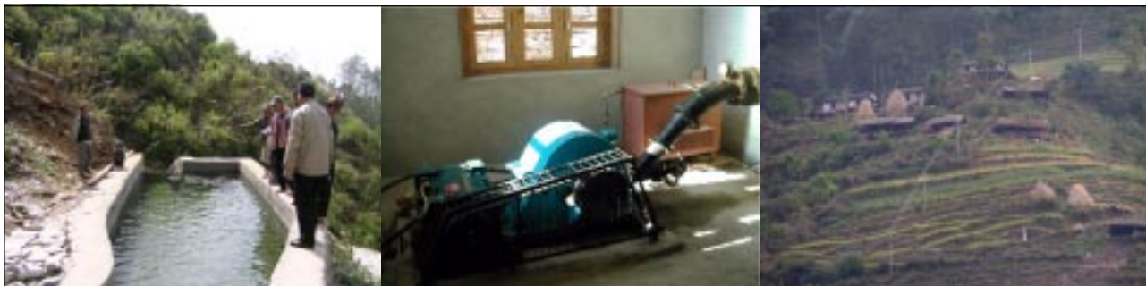
Figure 5: Micro-hydropower project – a forebay (left); turbine generator (centre) and power transmission lines across hilly terrain (right)
